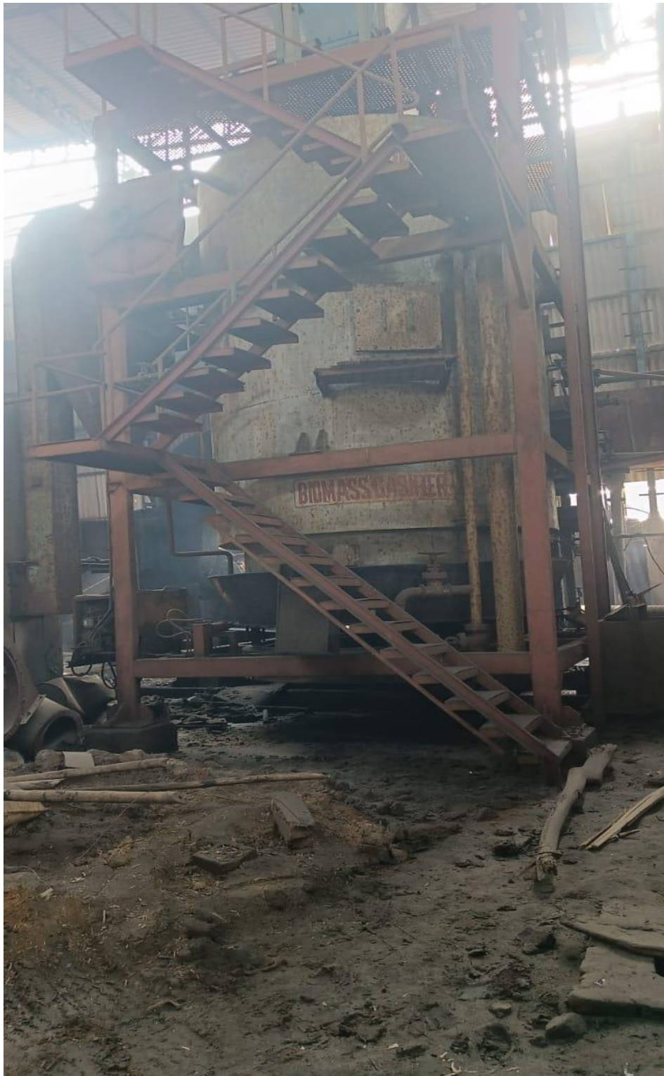
The Unit is having Biomass Gasifier
