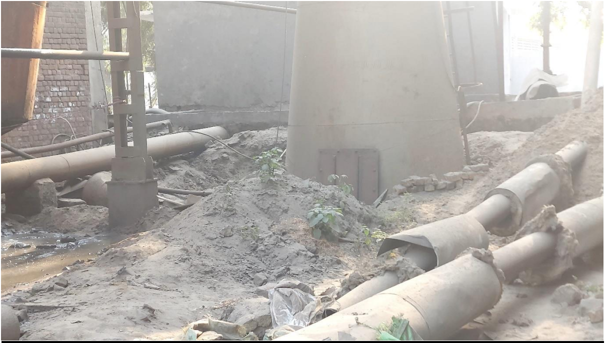
Fly ash was lying all around the Boiler suggesting improper disposal.
